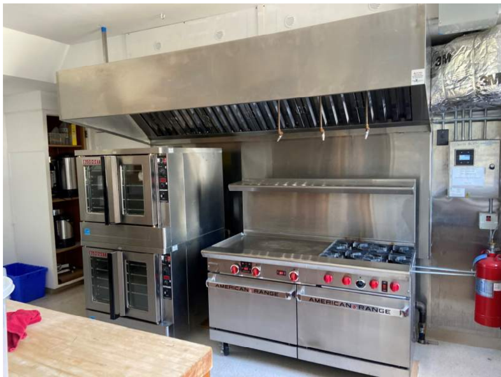
New 2019 Kitchen Equipment; Range/Griddle, Oven and Hood Assemblies
