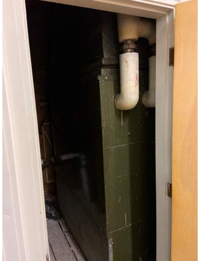
Sanctuary AHU in Dedicated Closet
