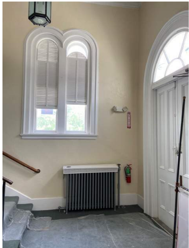
Entry Area Cast Iron Steam Radiator
