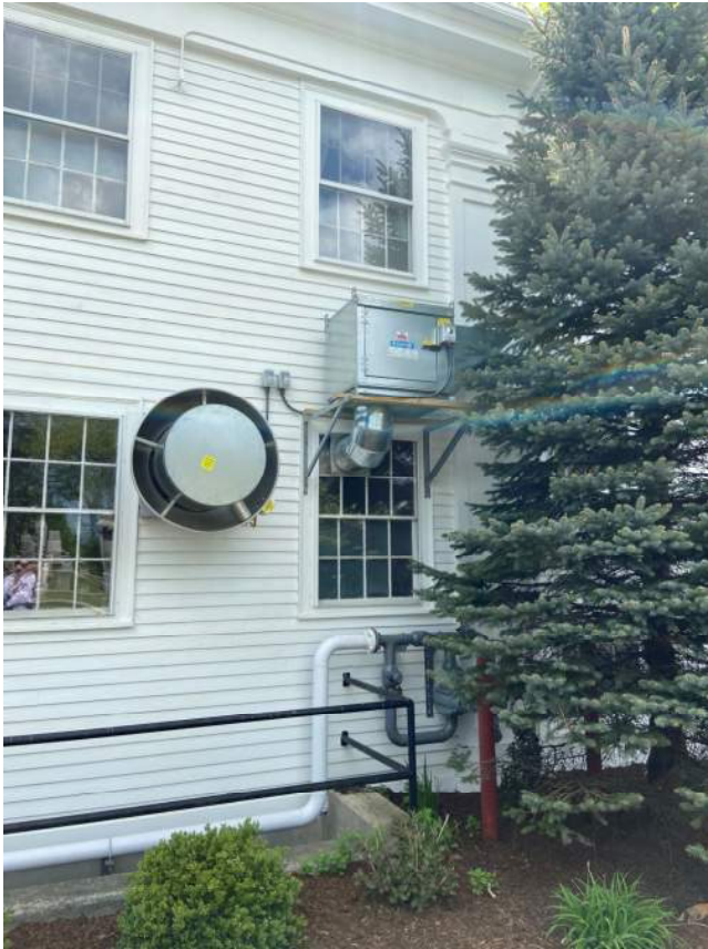
New Kitchen Exhaust Fan and MAU
