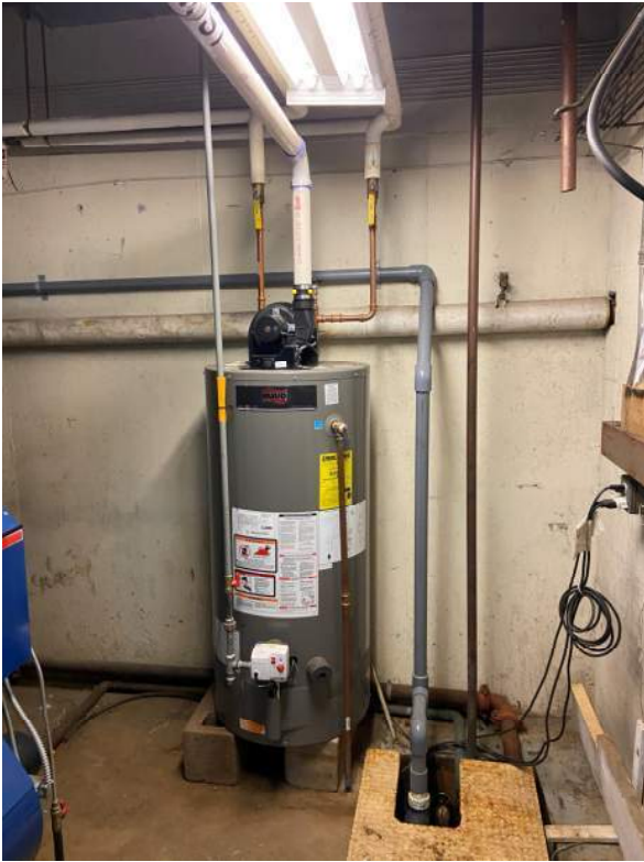
DHW Gas-Fired Heater System 36MBH
