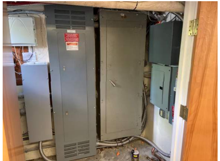
Electrical Service Panel and Solar PV Equipment
