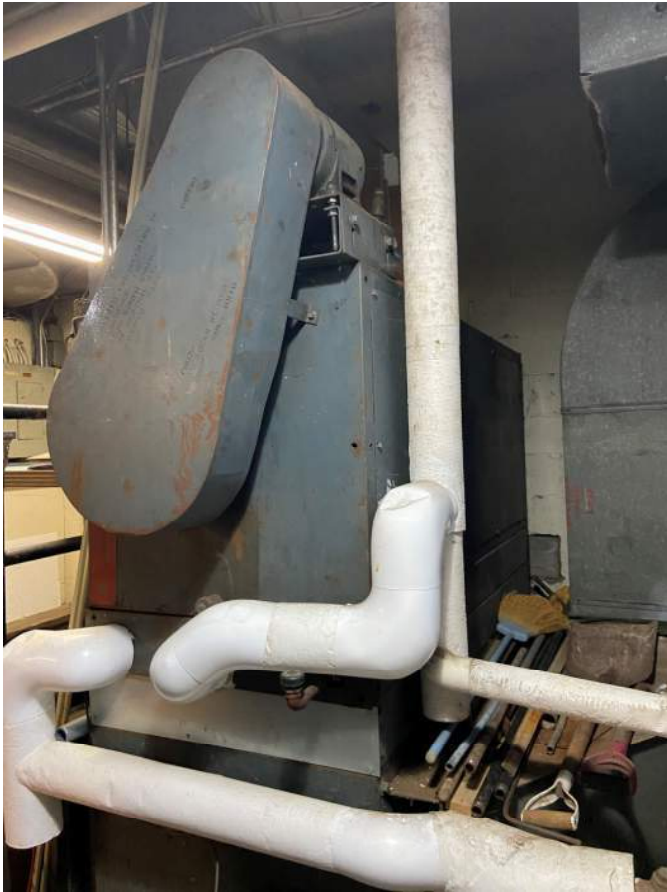
Fellowship Hall Air Handling Unit
