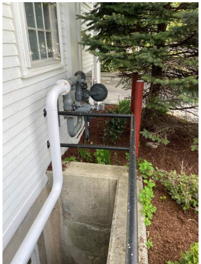
Gas Meter and Regulator Valve Assembly
