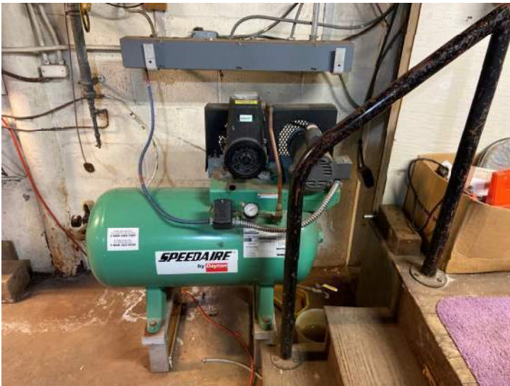
Air Compressor Serving Pneumatic Control
