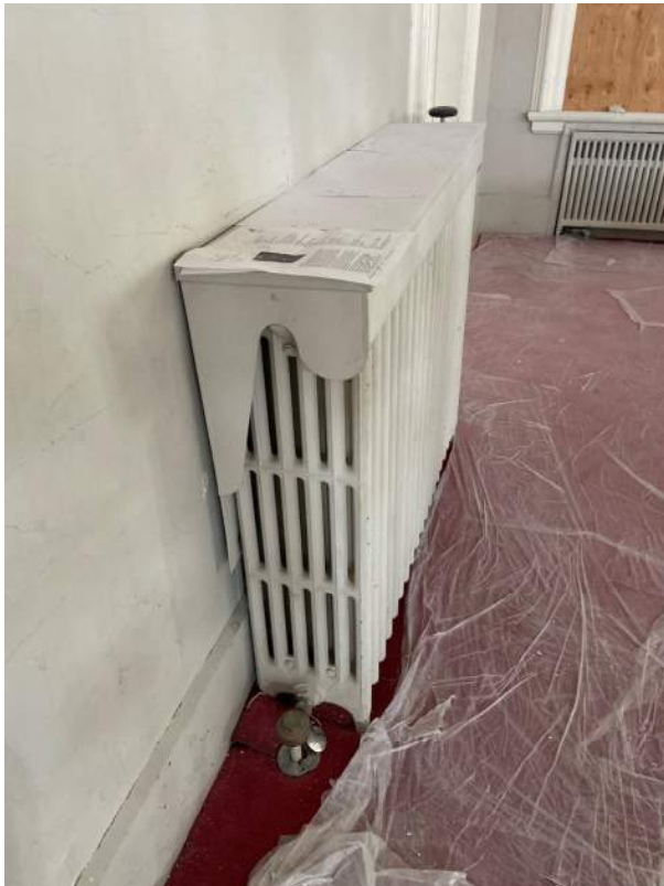
Sanctuary Typical Cast Iron Steam Radiator
