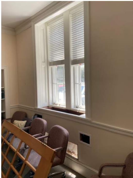
1860 Parish Room – Recessed Convectors
