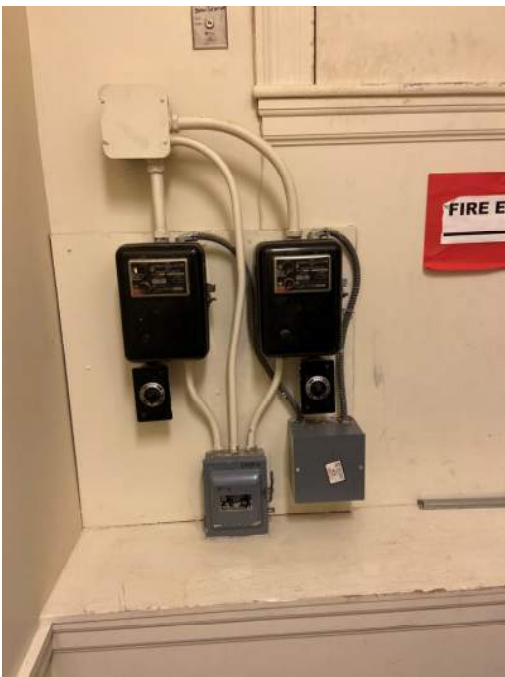
Sanctuary AHU Controls
