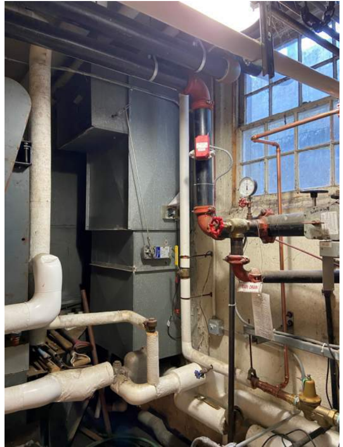
Boiler Combustion Intake & AHU OA Intake Louver
