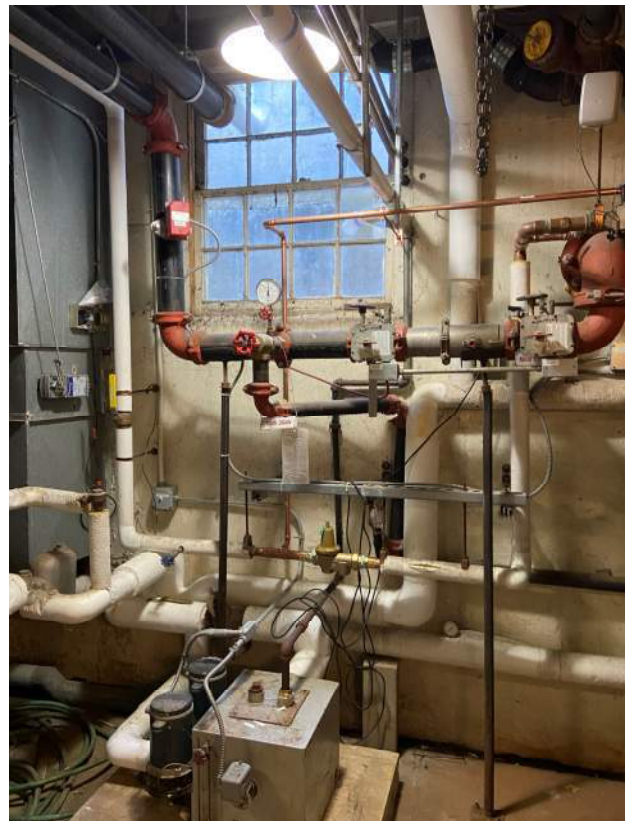
Condensate Feed Pump & SPR Piping
